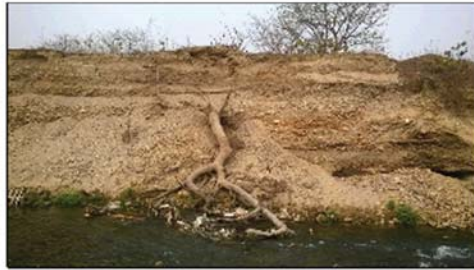
Plate 5. Exposed bank with coarse and loose particles at Dagapur Tea Garden susceptible to soil erosion
