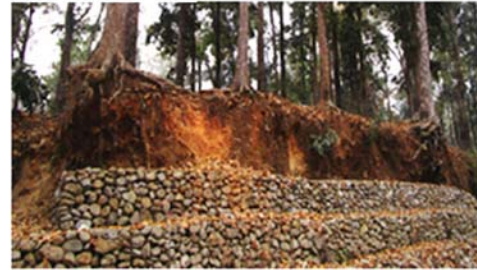
Plate 6. Erosion prone oxidised bank sediment at Sukna with three tier boulder wall
